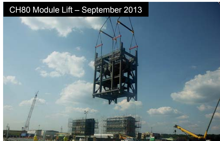
Photos © 2013 South Carolina Electric & Gas. All rights reserved.
