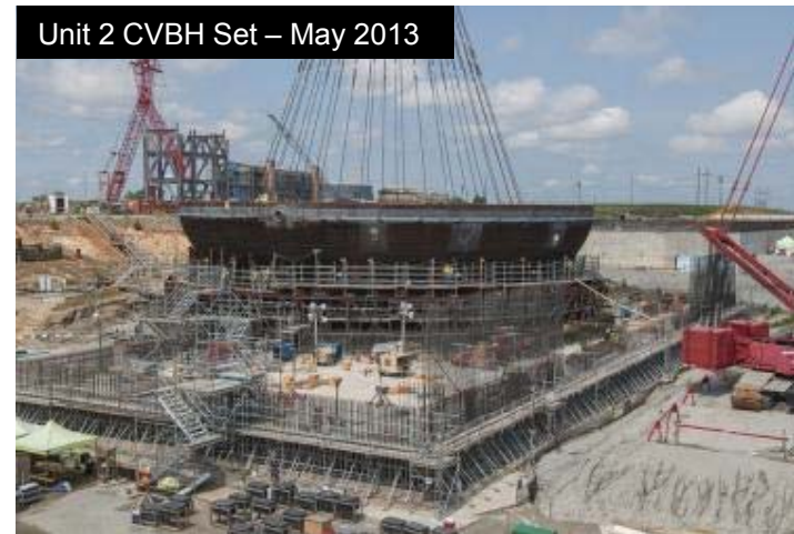
Photos © 2013 South Carolina Electric & Gas. All rights reserved.
