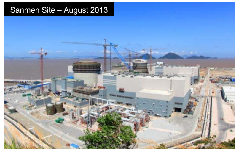
Photo © Sanmen Nuclear Power Company, Ltd. All rights reserved.
