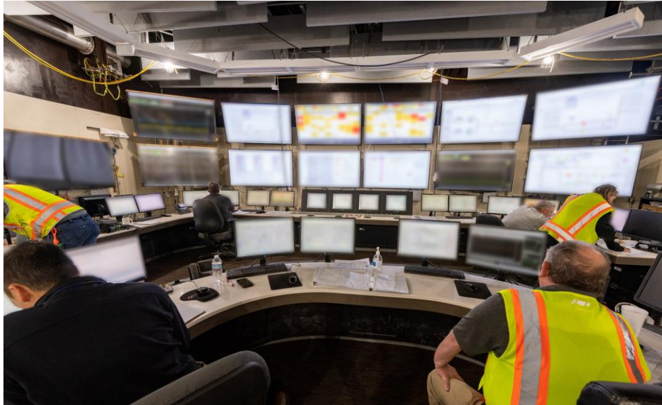
Left: Operating the Plant from the Main Control Room
